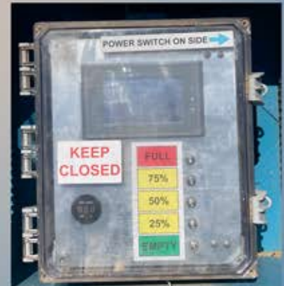
ELECTRICAL BOX INTERIOR
